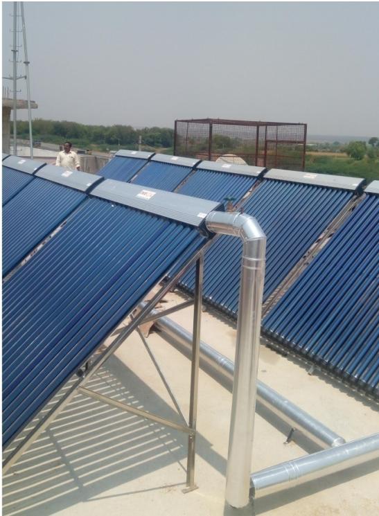
Solar Water Heater
